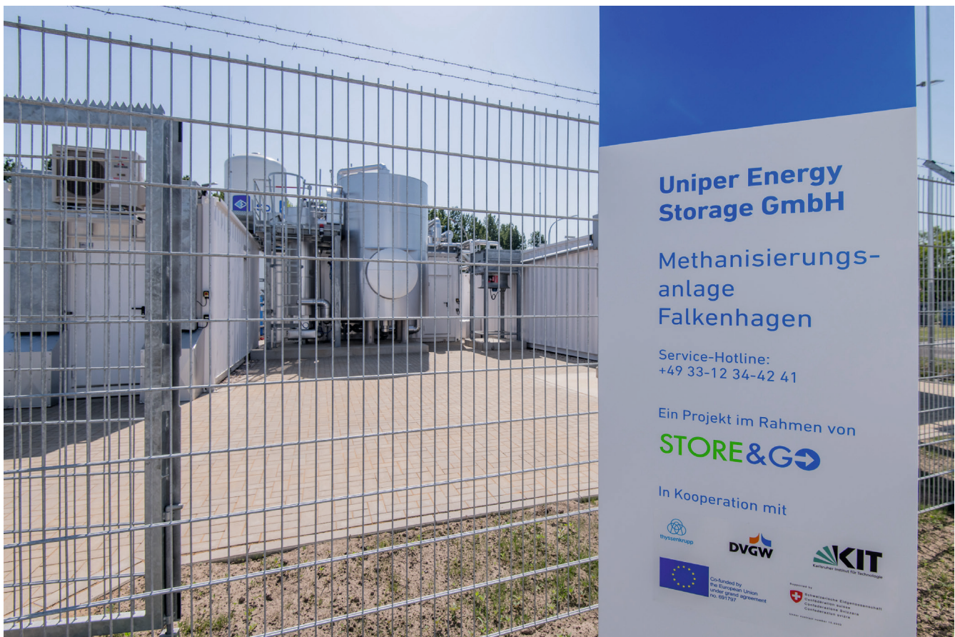
Figure 02: Methanation plant in Falkenhagen
