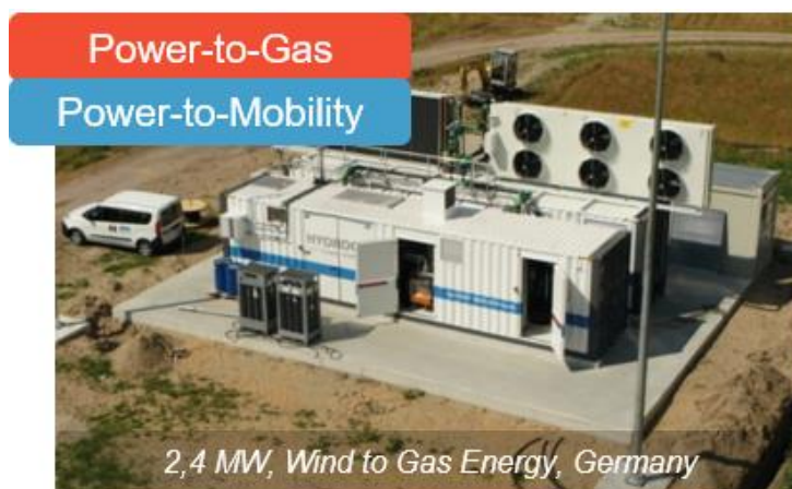
Figure 1: 2.4MW PEM electrolyser in Germany
